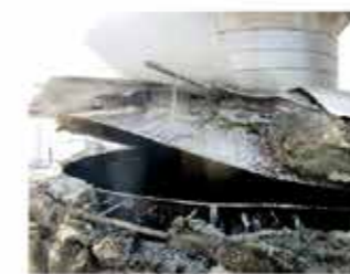
Converter roof open like dolphin fish mouth
